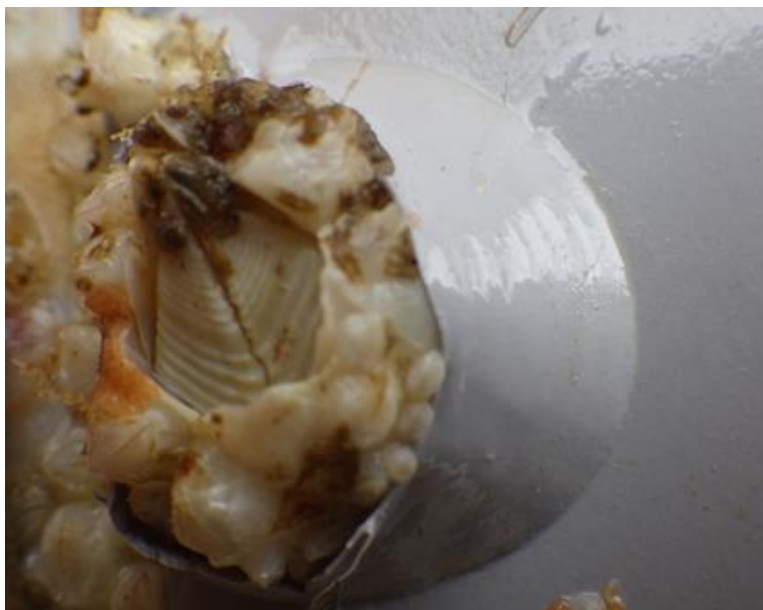
Figure 8: Coating damage caused by growth of a barnacle
