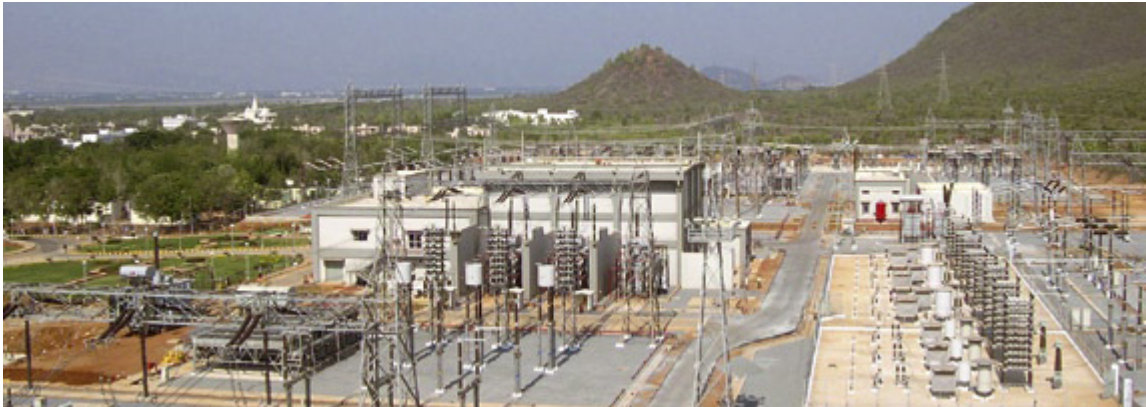
Fig. A9: Converter station of the 500MW Vizag II LCC-HVDC system connected in back-to-back configuration with \pm 88\text{kV} DC link voltage (source: ABB website www.abb.com )
