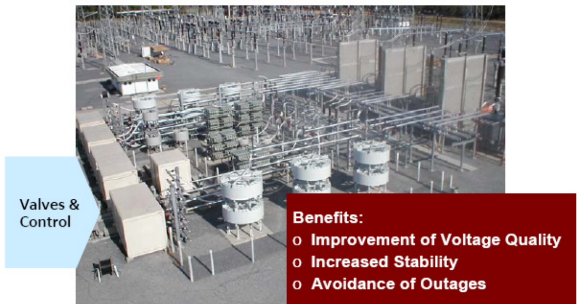
Fig. A3: SVC Bom Jesus da Lapa, Enepower, Brazil-500kV, \pm 250 MVar reactive power capability [78,104] (Source: Siemens website)
