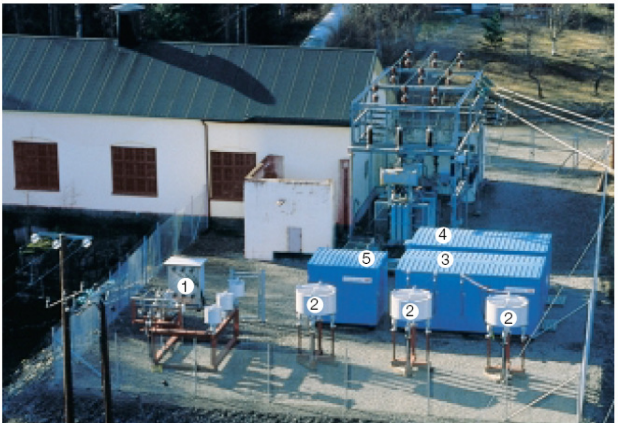
Fig. 10: HellsJÖn test installation in Sweden. The world's first HVDC Light transmission link rated at 3MW with bipolar DC link voltage of \pm 10\text{kV} , using 10km decommissioned AC line (for demonstration purpose). (Source: ABB website www.abb.com )
