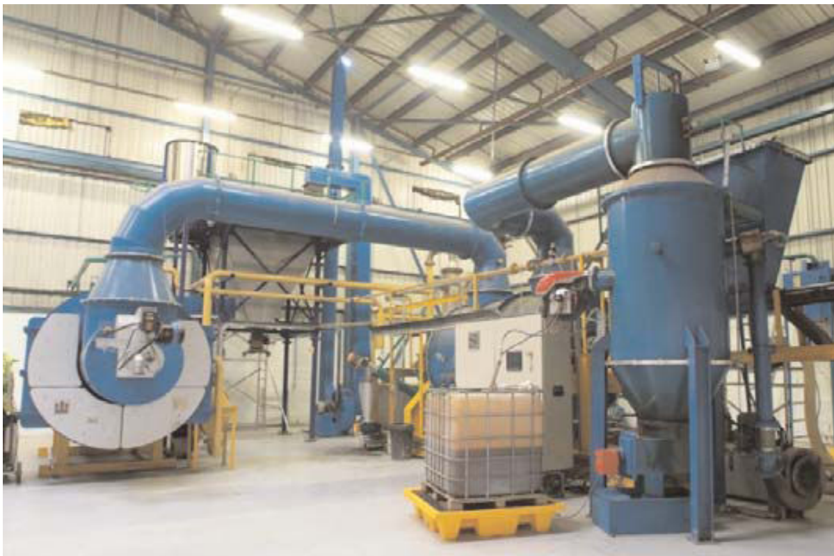
Figure 12: Stein demonstration plant in Rotherham (courtesy of First Power Ltd)
