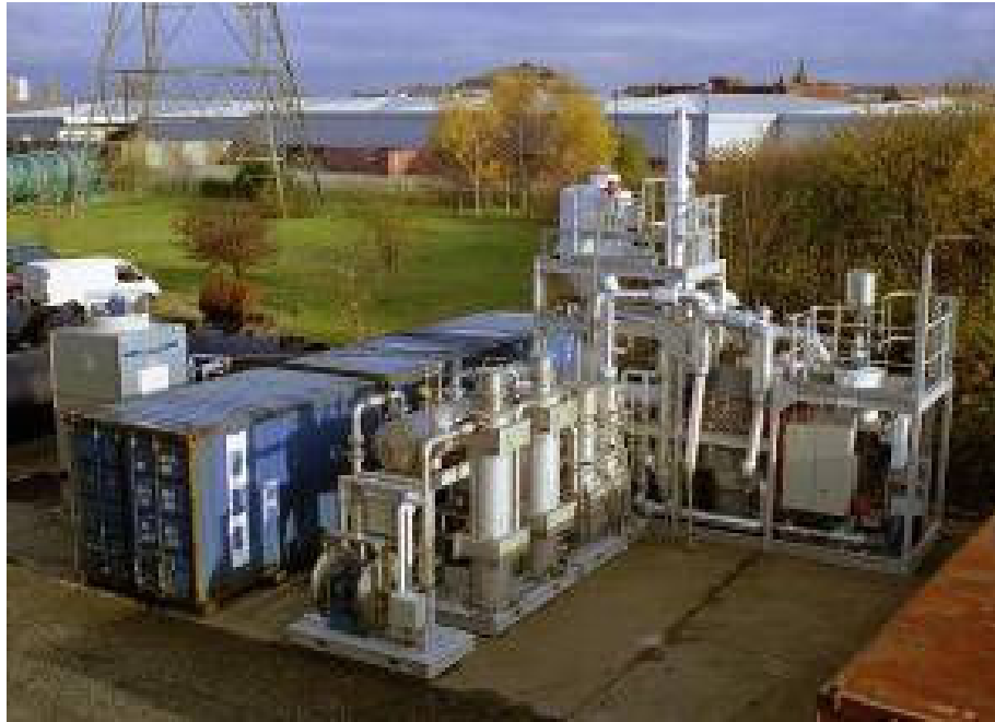
Figure 20. 250 kg/h fast pyrolysis plant, Oldbury
