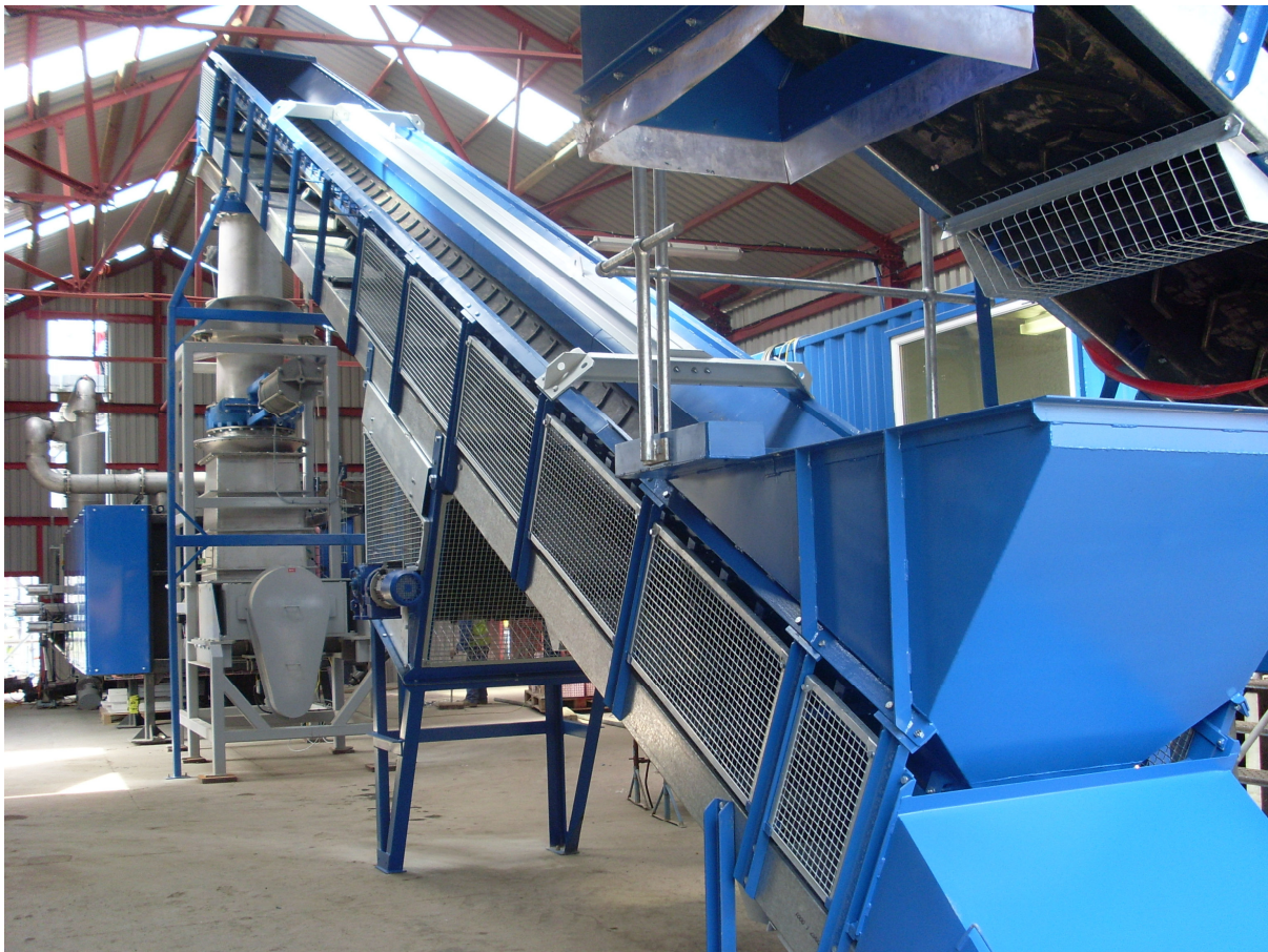
Figure 12. EPI plant, Mitcham
