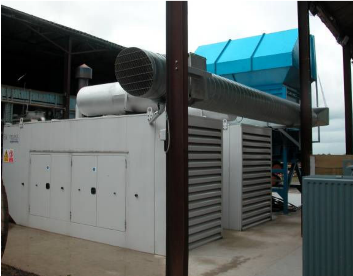
Photograph 5. Iveco gas engines in acoustic enclosures and exhaust gases dilution fan and duct
