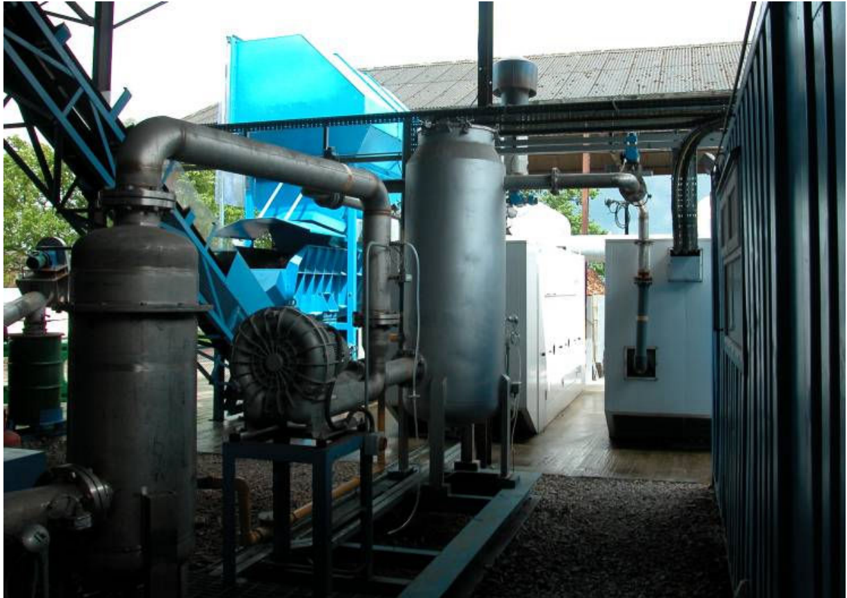
Photograph 4. Demister, Gas fan and Gas buffer tank [engines in background]
