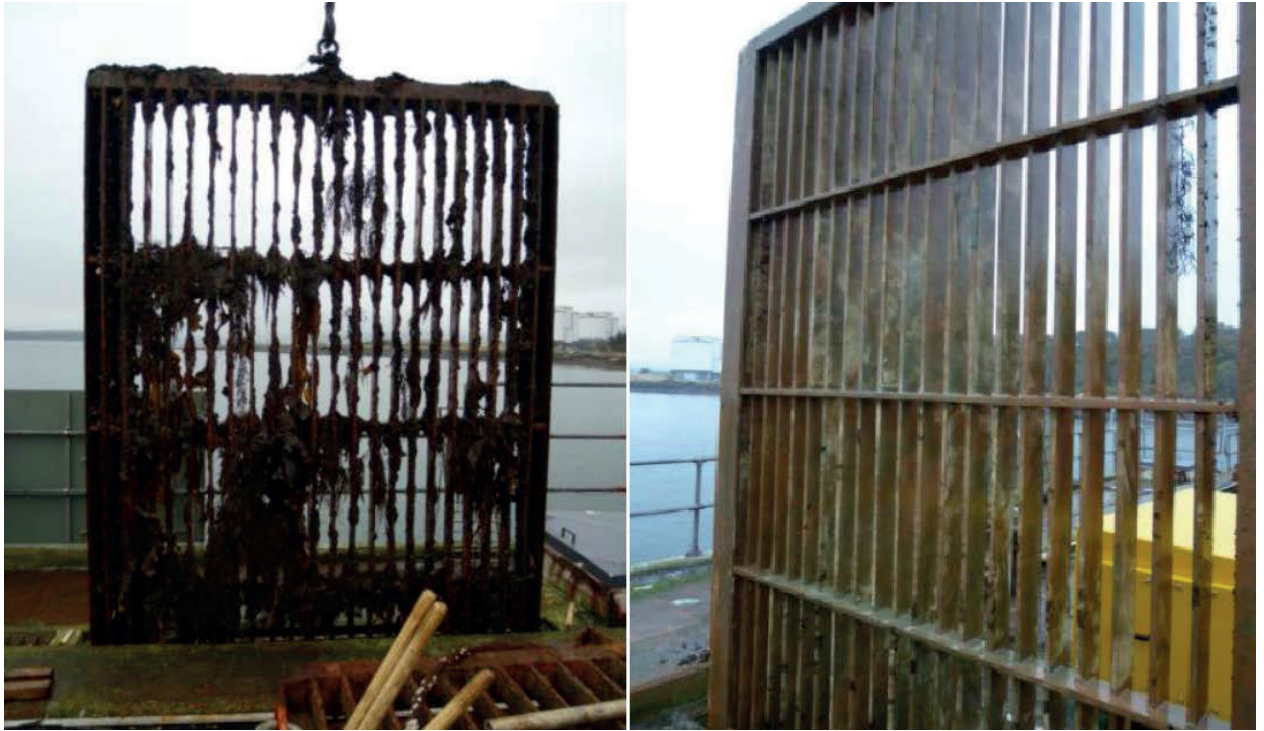
Figure 2. HNB coarse screens after five weeks in situ during normal operation. Screen with new coating on the right; untreated screen on the left. (Source: EDF Energy)
