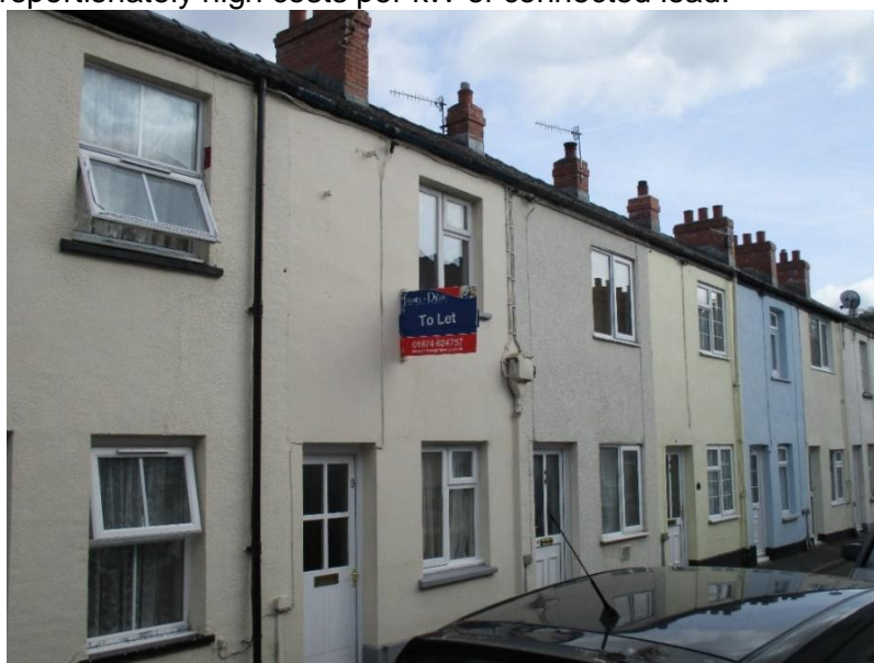
Figure 15: Typical pre-1919 terraced housing – note electricity distribution is external at eaves level from junction box on wall
