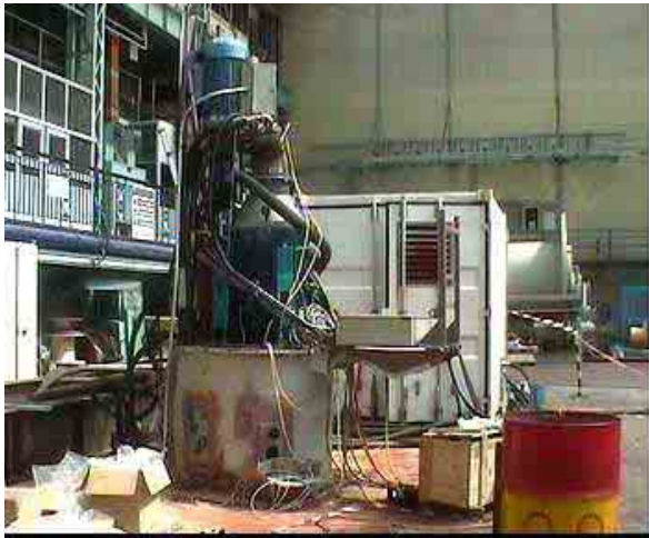
Figure 6: Pod contents (main motor at base, auxiliary motor at top), with hired in HPU in background
