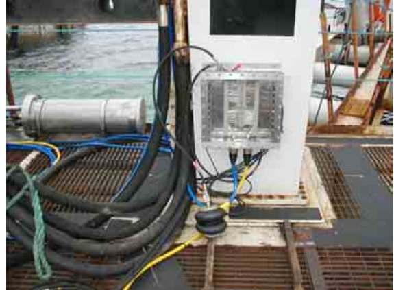
Figure 3: Instrumentation Pod and Junction Box in position on Stingray
