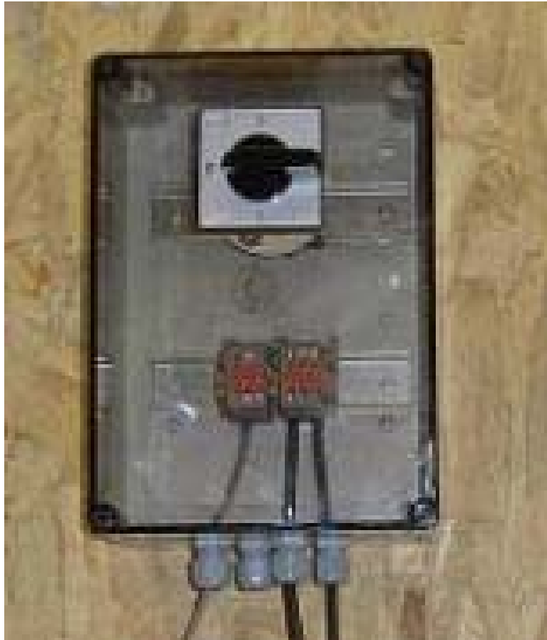
Fig BF. Marshalling Box..
