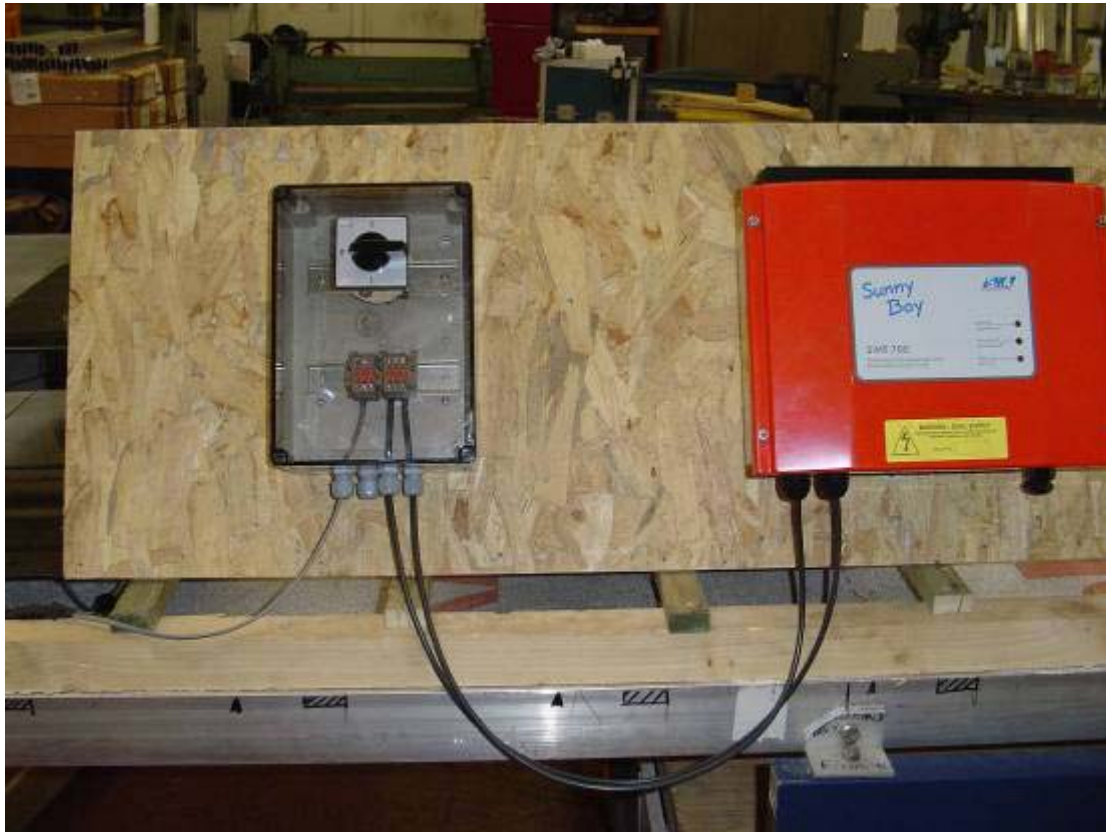
Fig BG. Inverter connection.
