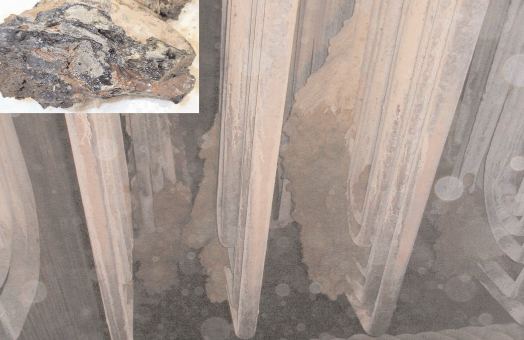
Figure 1. Example of slag build-up in a power station boiler
