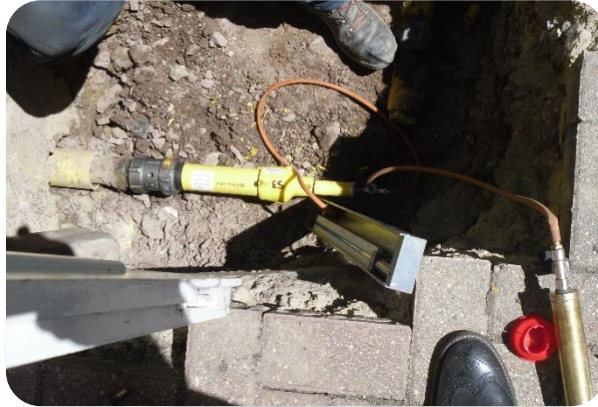
Figure 11: Pressure test on the installed Serviflex pipe at the outside connection point.
