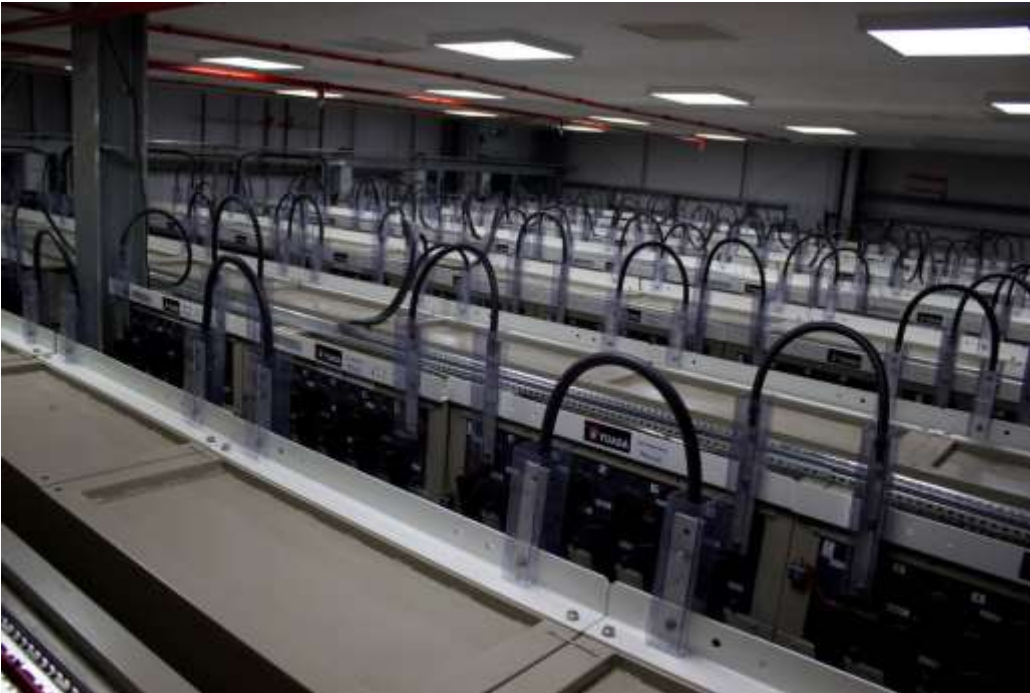
Figure 27 - Installed battery (i)
