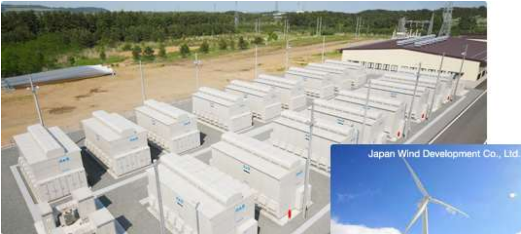
Figure 1 - 34MW NAS battery
