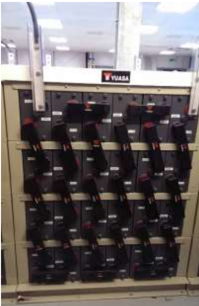
Figure 24 - VRLA battery rack
