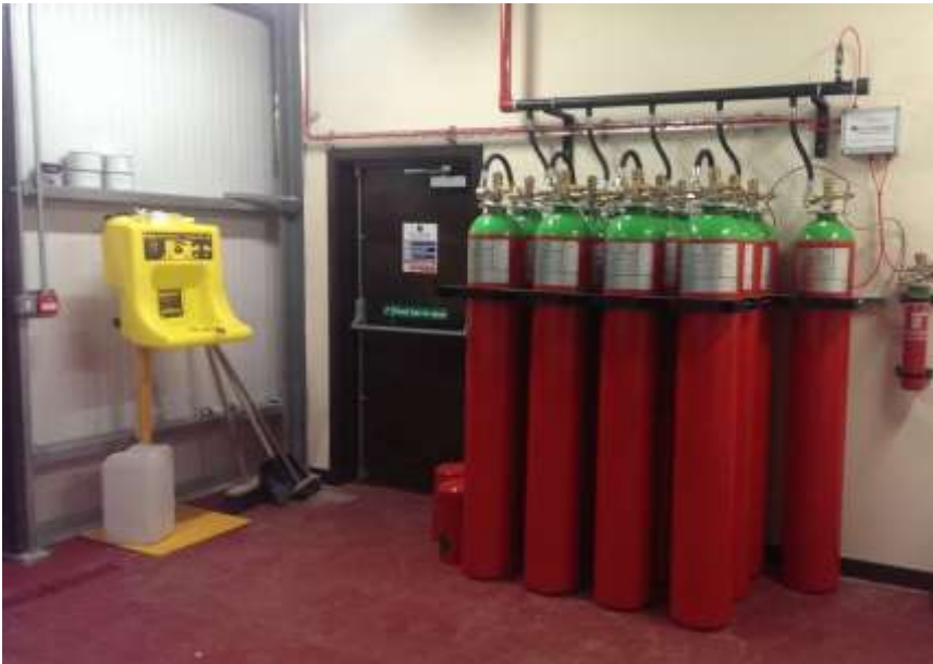
Figure 31 - Inert gas for fire suppression
