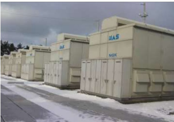
Figure 5 - 34MW battery, Rokkasho wind farm, Japan
