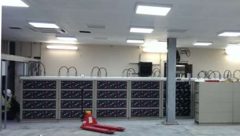
Figure 23 - VRLA battery installation
