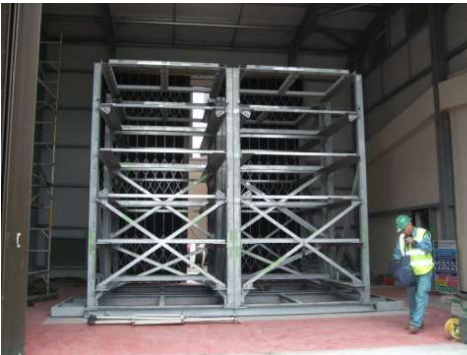
Figure 11 - Installed battery enclosure frame
