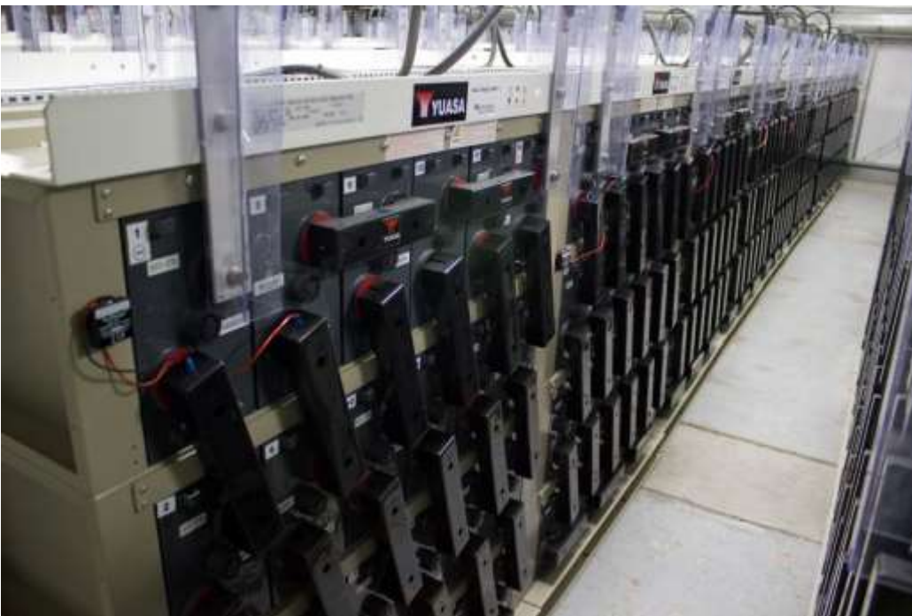
Figure 28 - Installed battery (ii)
