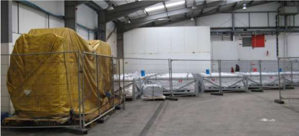
Figure 10 - Battery modules and PCS in storage on Shetland
