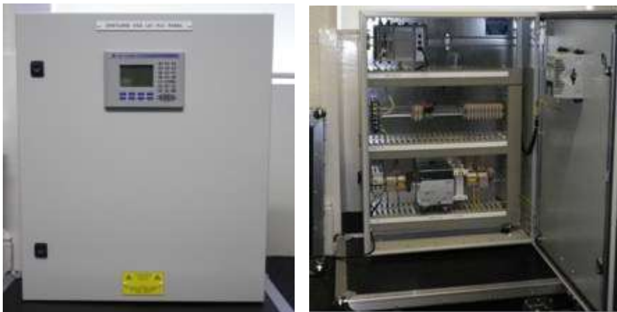
Figure 19 - Local interface controller
